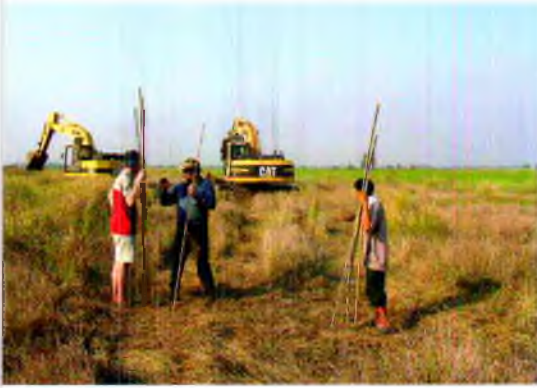
The edges of the letters are marked with poles, so that work with the excavator can begin.
