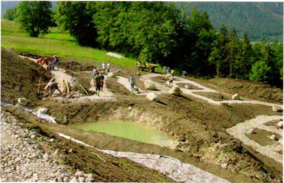
The structure of the sensory garden: the remaining work mostly needs to be carried out by hand.
