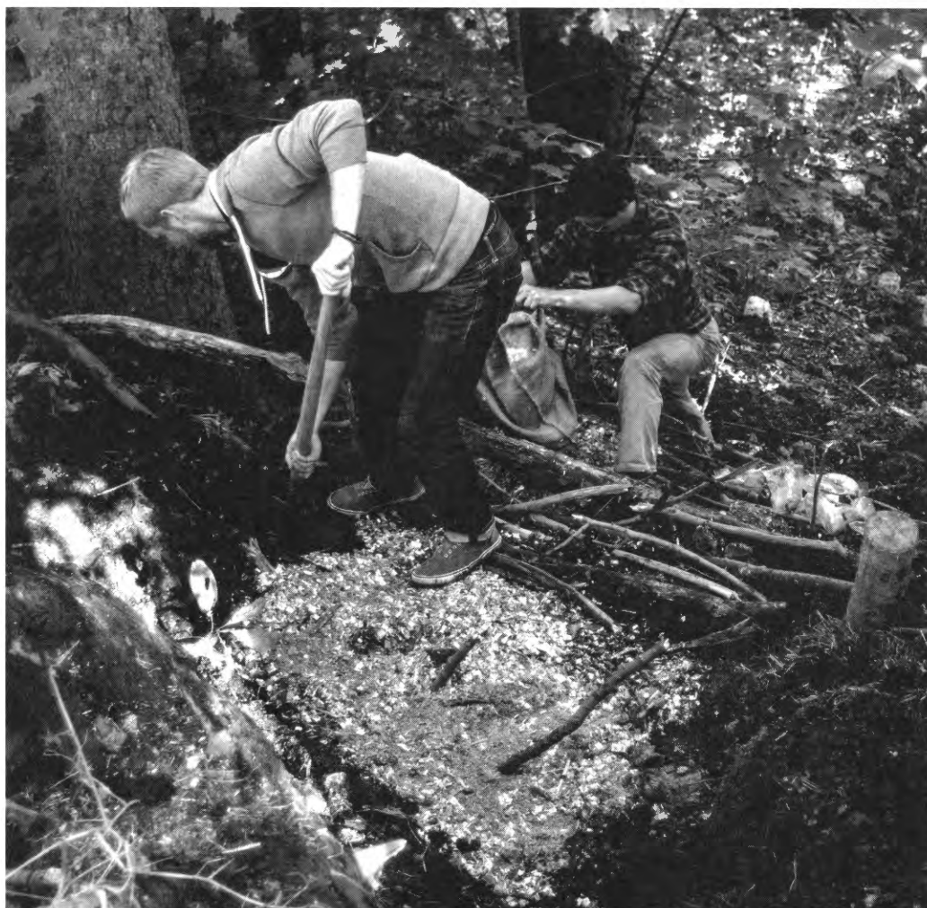
A two-tiered microbial filtration system, designed by the author, being installed in western Massachusetts. The target pollutant was effluent overflowing from an antiquated septic system.
