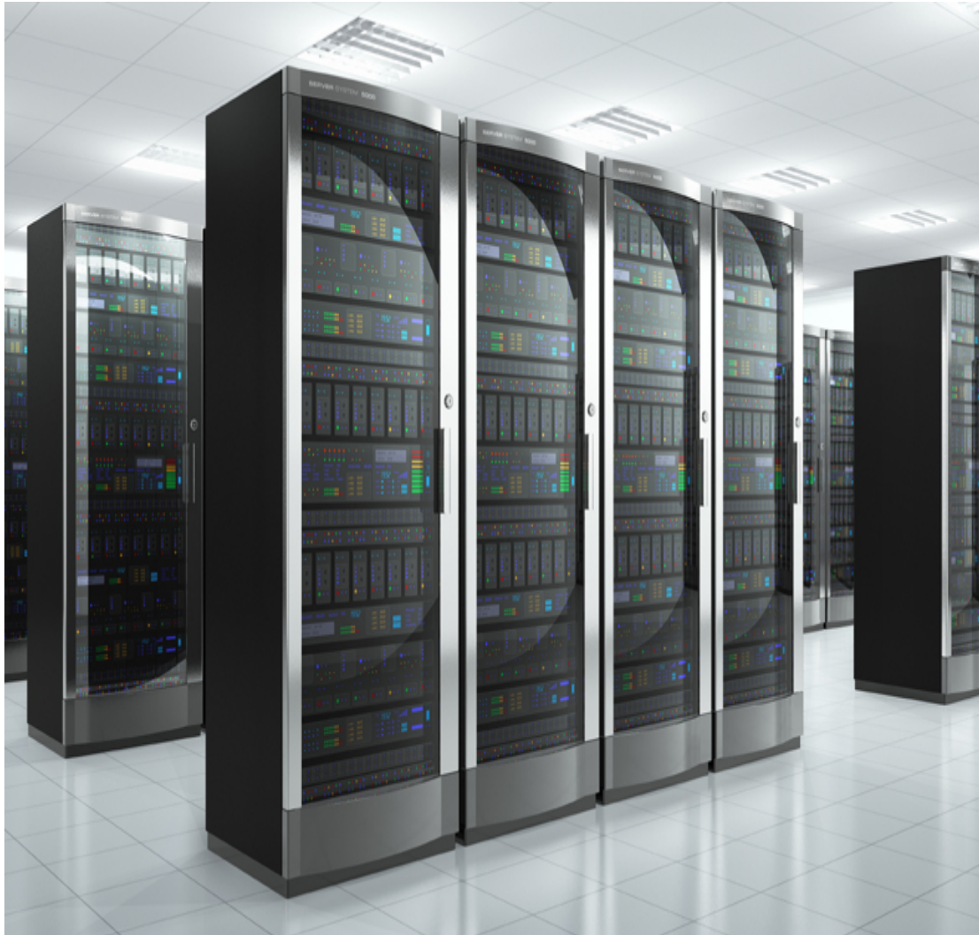
Figure 17.1 A cloud data center
